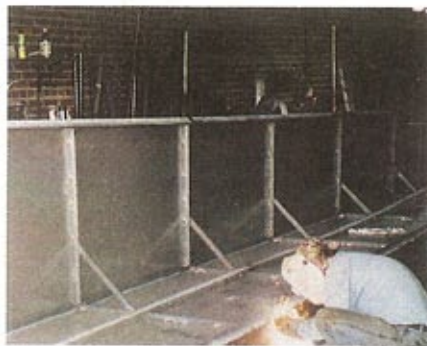
Fig. 1 — Welding sides one and two together. Carbon steel bars were used to reinforce the corners.
